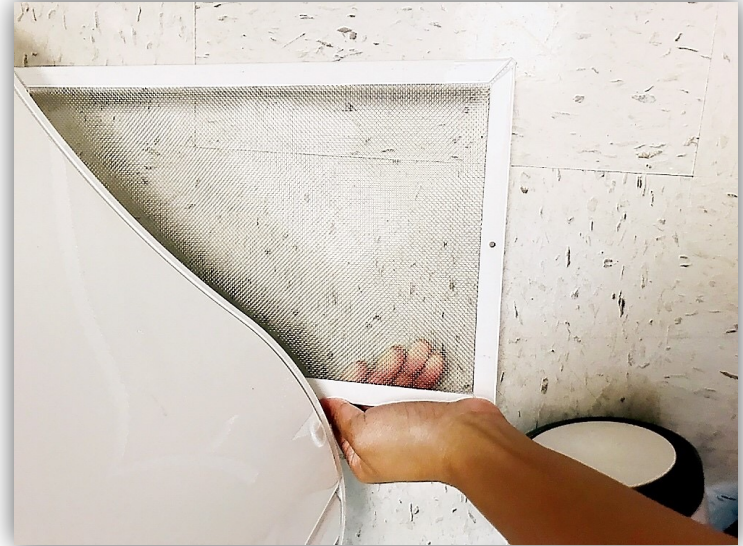
Image above: fan screen located under console (magnetically attached)
